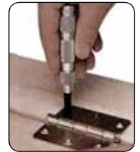
Punch being used to mark screw starting centres on a door frame
